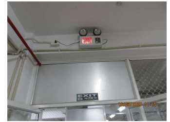
Exit mark & emergency light.JPG
