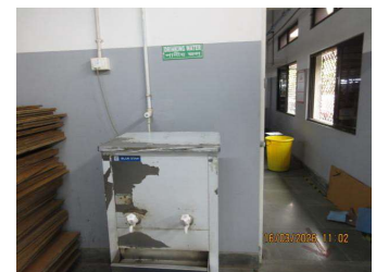
Drinking water point.JPG
