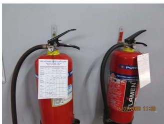
Fire extinguisher inspection records.JPG
