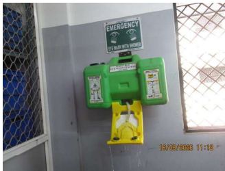
Eye wash station.JPG
