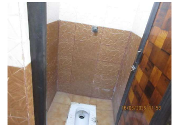
Female toilet- inside.JPG
