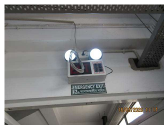
Emergency light working.JPG
