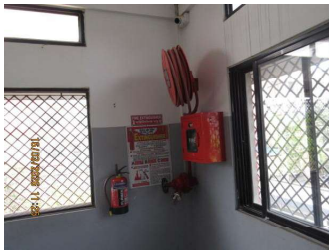
Fire hydrant & hose reel.JPG
