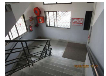
Staircase with hydrant-hose reel.JPG
