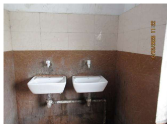
NC- No handwash soap in male toilet.JPG
