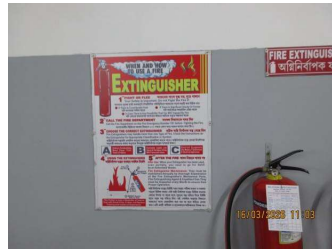
Fire extinguisher operating instruction displayed.JPG
